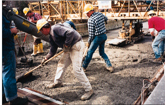
Drivers should warn workers when they see causes of cement burns, such as failure to wear tall rubber boots.
